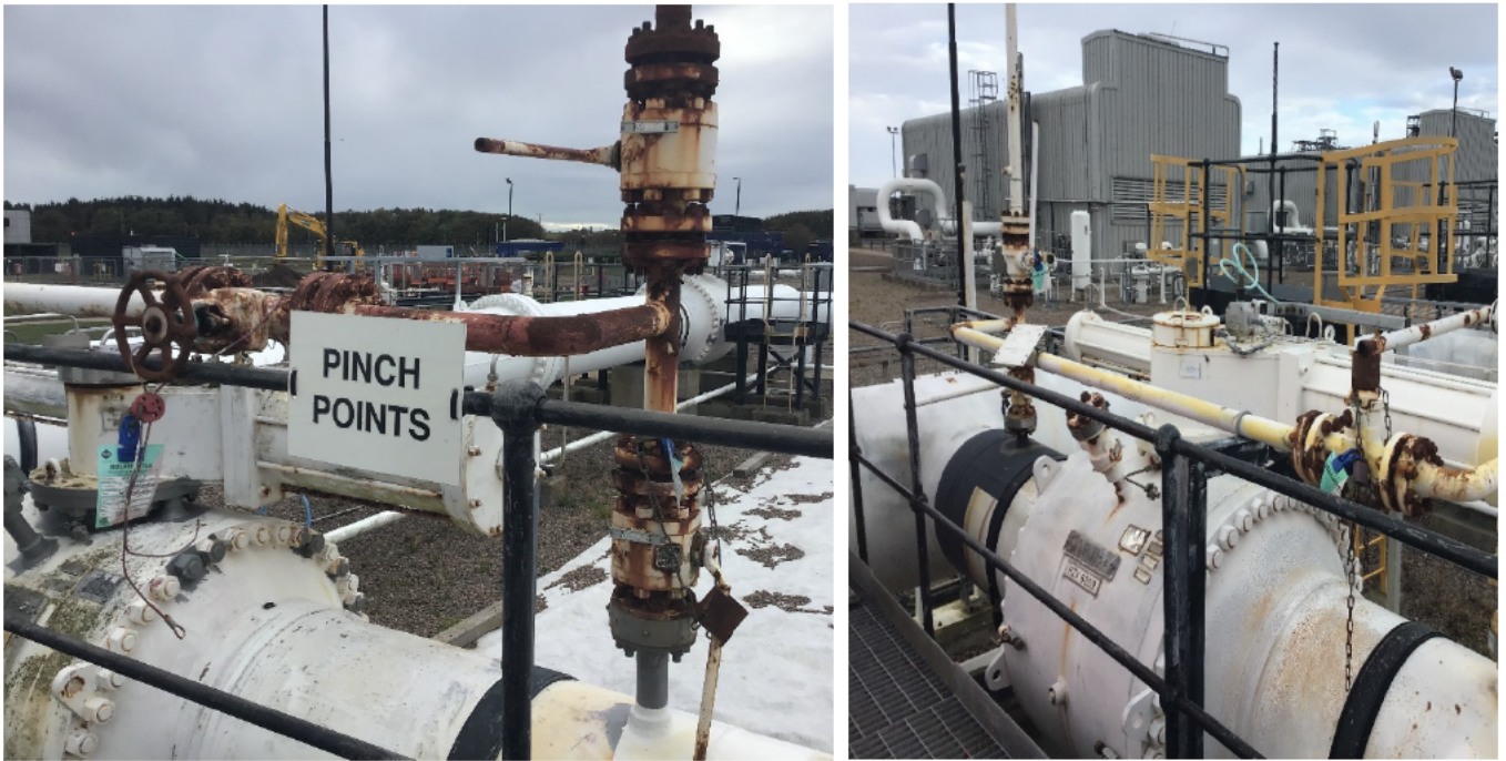
Figure 7 Category 6 corrosion defects on above ground pipework in the mixing area (located in area 6) of the terminal
